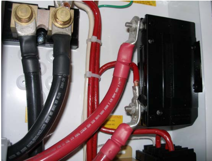
Battery Positive connections and shunt wiring
